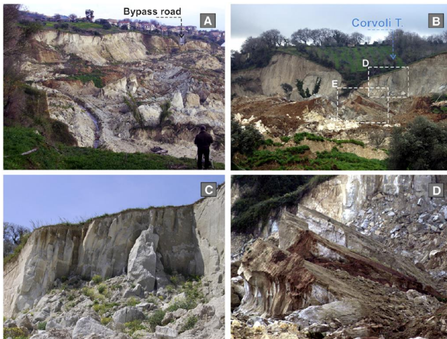
Figure 4.10 – Photos taken in the upper sector of the landslide: (A) main scarp (about 600 m) that extends from NE to SW, making a gentle curve; (B) valley of the Corvoli Torrent that split the main scarp into two parts; (C) bands of parallel joints (about 15 m wide), NE-SW trending, related to the decompression that occurred during the landslide movement along the main scarp; (D) large rock blocks rotated backwards. (From Borrelli et al (2014))
