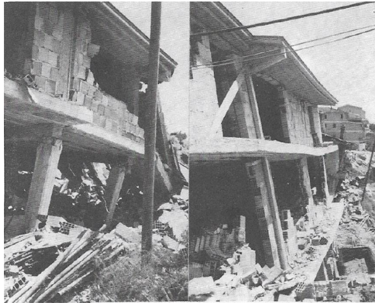
Figure 3.6 – Building 11, clearly damaged and carried downwards from the landslide for about 15 m (from Viggiani & Di Maio (1991))
